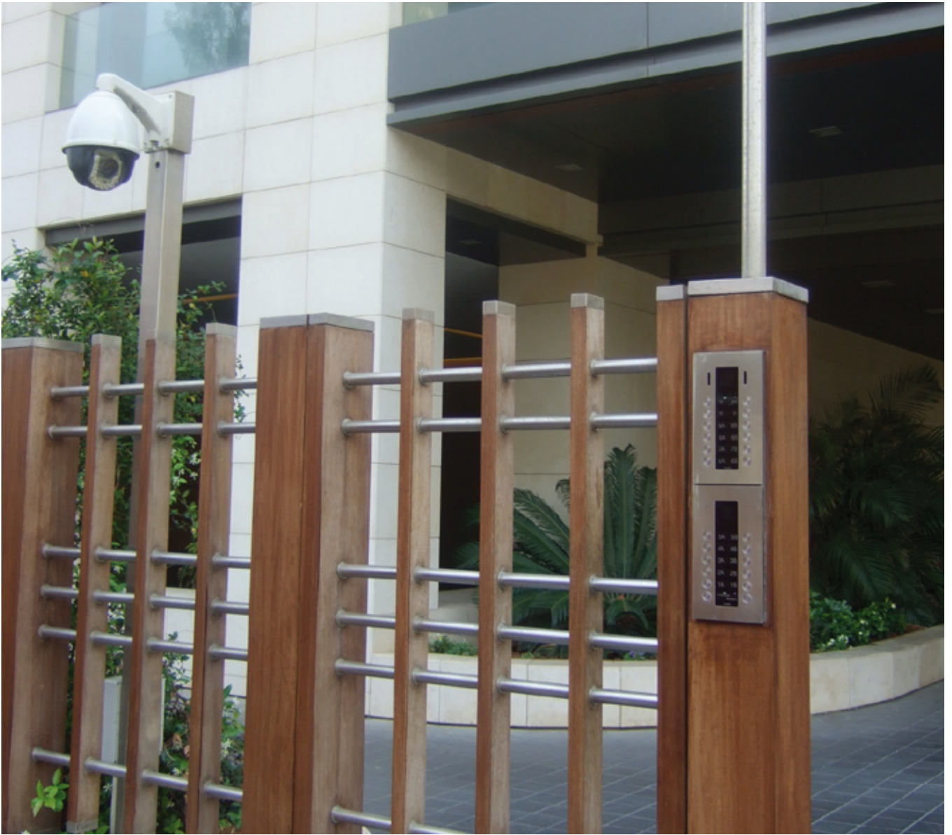
Tactile Monitors & Alea entry panels in Qoraytem Bldg. (Lebanon)
